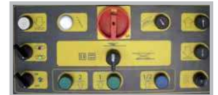
• Quadro comando • Control panel
